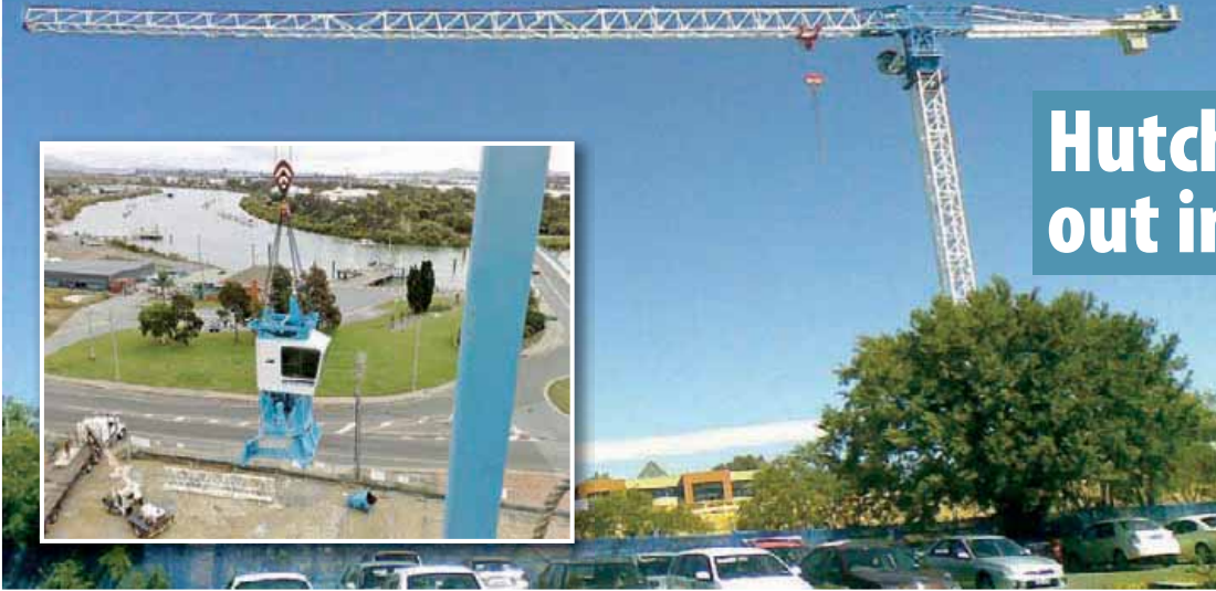
Hutchies' Crane and Hoist team is now providing cranes and hoists to other builders throughout Australia.
